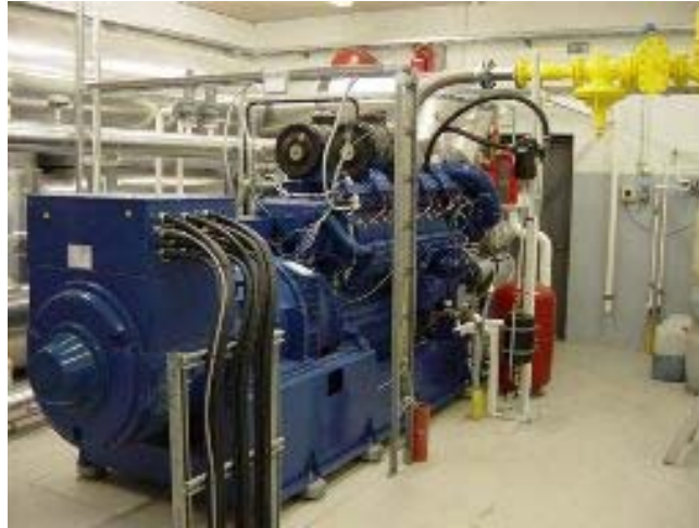
Figure 3 A 16 cylinder 35 litre gas engine used to produce electricity in Alvik
