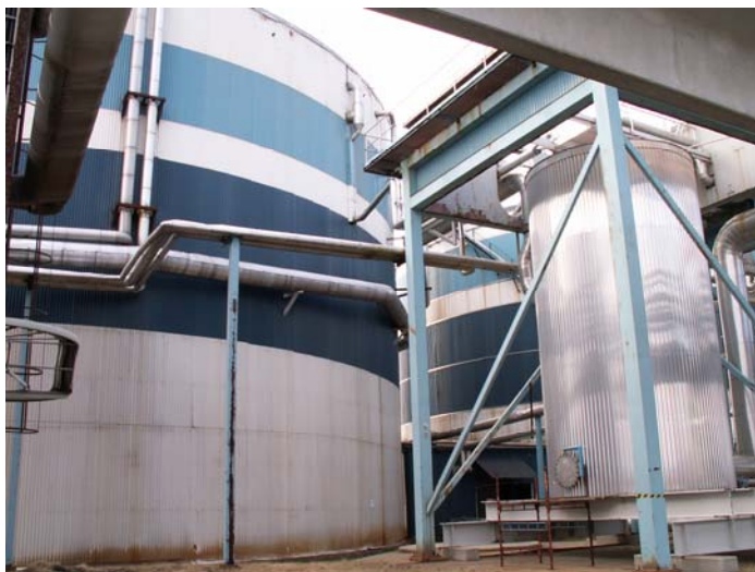
Figure 1 The biogas plant at Domsjö. The blue and white tanks are anaerobic digesters and the polished steel container is a de-gassing tank.
