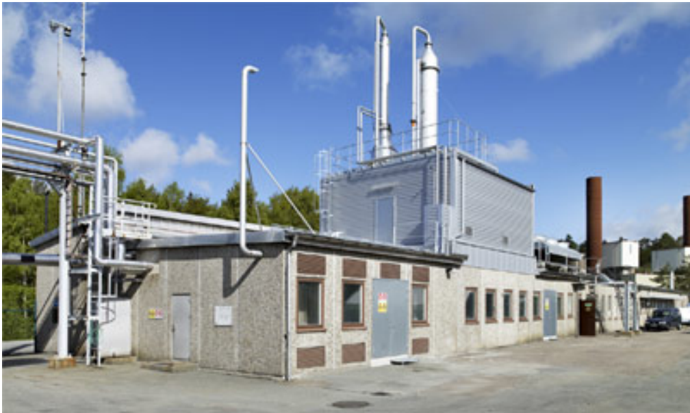
Figure 1 The upgrading plant at Arendal, Gothenburg
